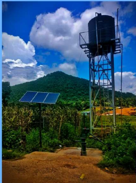
Photograph No: 5.2 Water supply system run by soller
